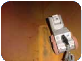
Remote visual inspection of service water piping systems for MIC using robotic crawlers and high-resolution video cameras.
