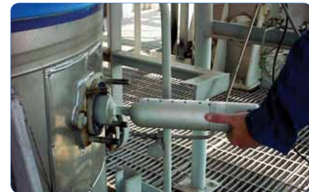
A PTZ camera system is used to inspect the integrity of glass- and refractory-lined vessels.
