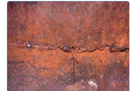
Weld defects can cause significant equipment inspection challenges
